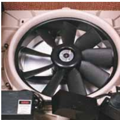
The inside of a Commercial Air unit
